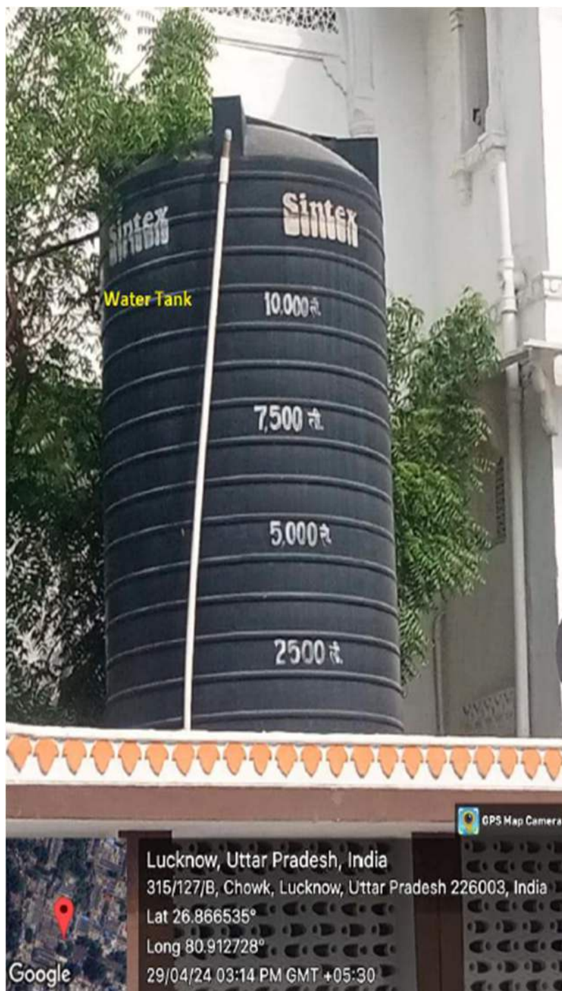
Water tank on roof top of hospital building
