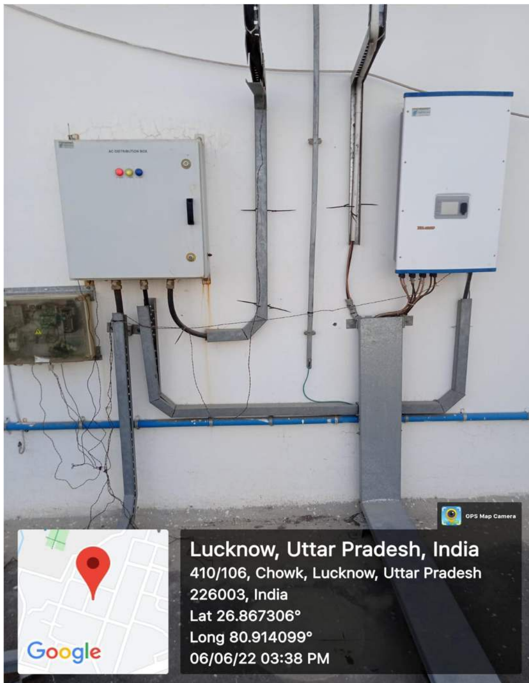
Wheeling to the Grid at Shatabdi Phase 1
