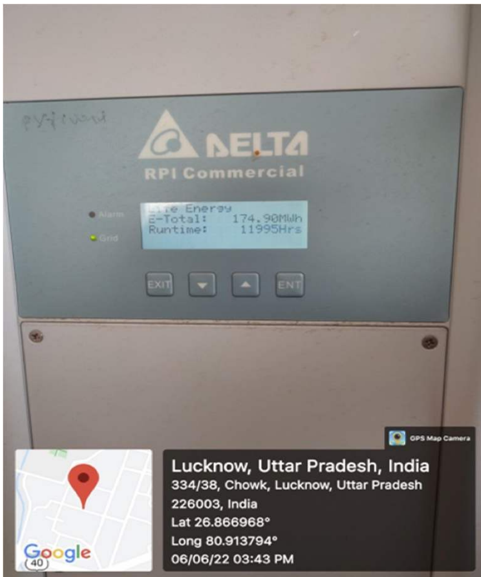
Wheeling to the Grid at old Administrative Building
